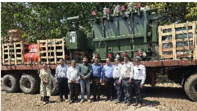
10 MVA Transformer Commissioned at Ambad Substation-3: A Major Boost for Power Infrastructure
